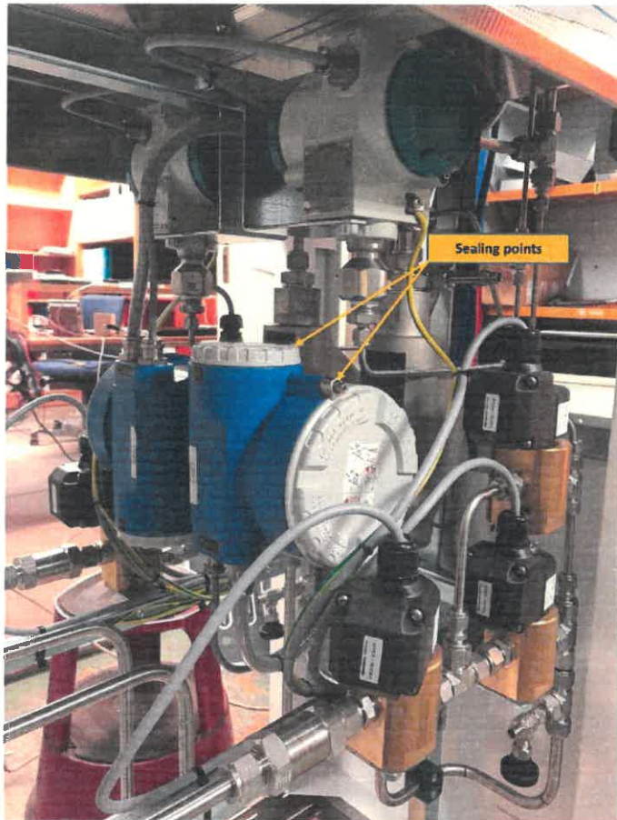
Figure 1: Sealing points of the measuring device
